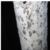
ACM- Pipe insulation (T.S.I)
