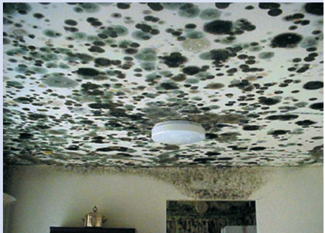
Photo 2: Extensive mold contamination of ceiling and walls
