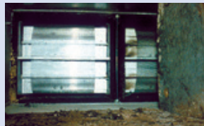
Photo 4C: Moldy air duct
