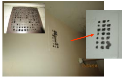
Covered or dirty grilles
