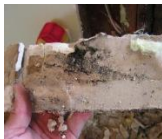
ACM- Spackle/Joint compound
