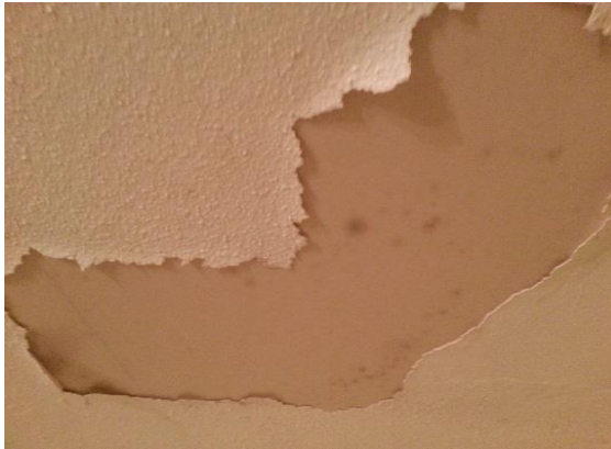
Bath room ceiling
