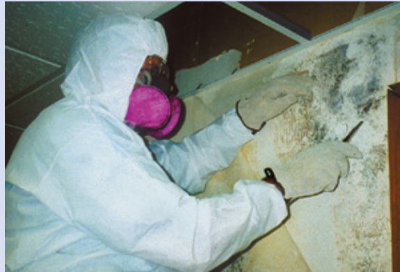
Photo 7: Remediation worker with limited PPE
